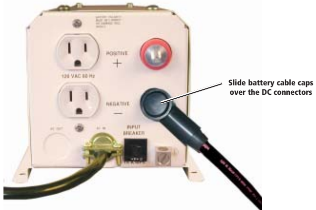
Figure 2-12 Battery Cable Caps
